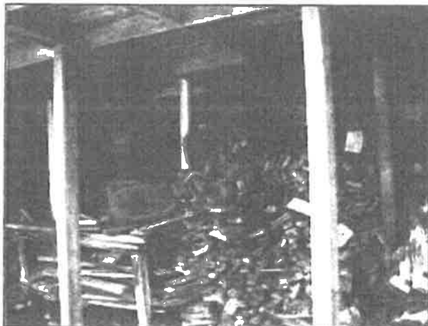
No deck, regardless of the material used to build it, would be safe if this amount of fuel beneath the deck caught fire. Even decks that may have a noncombustible surface, such as concrete, use lumber and timbers for structural support and those materials can catch fire.
